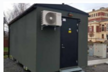
Technical spaces and cabinets
