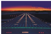
Airport Ground Lighting (AGL)
